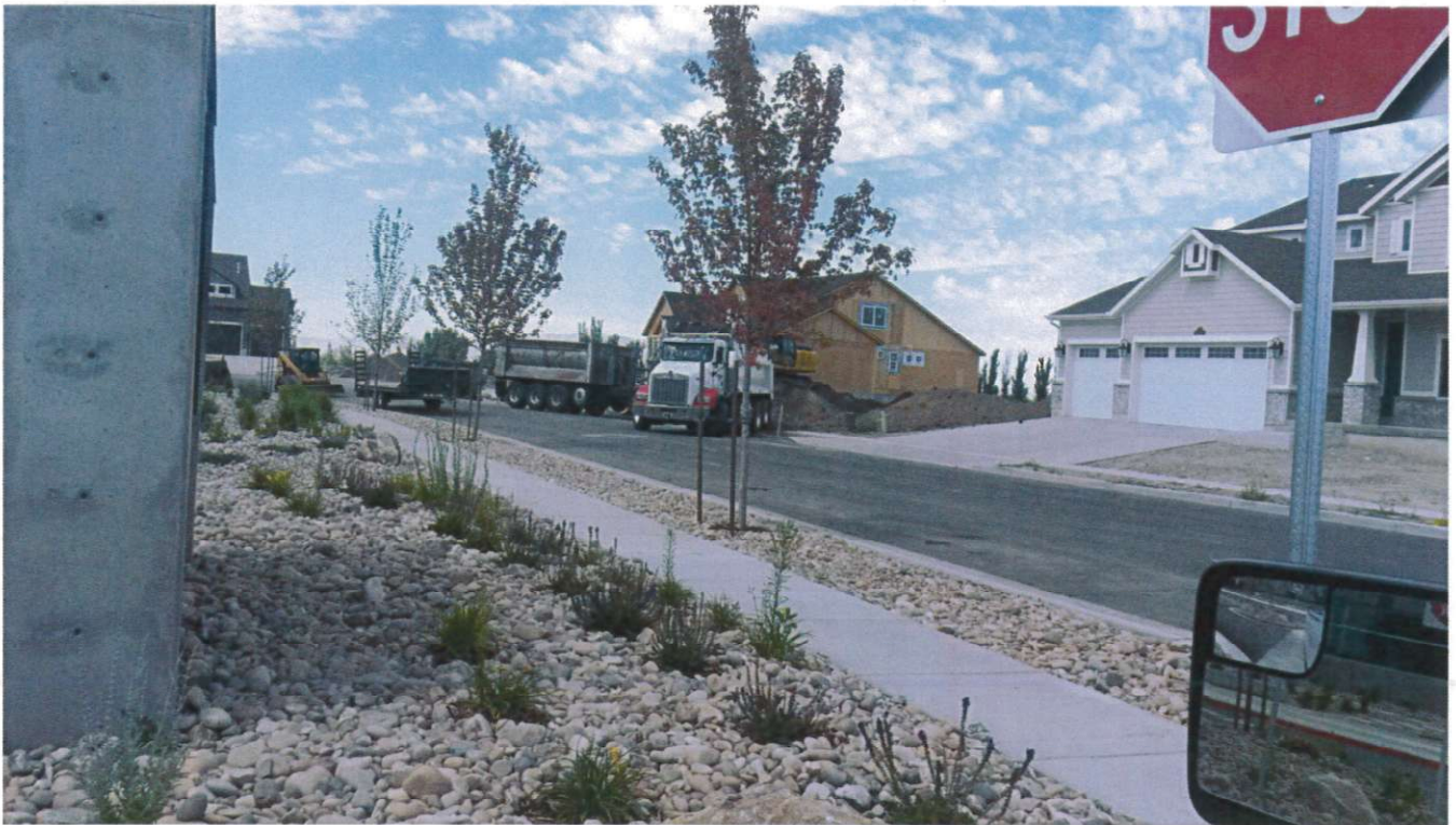
Photo 2: Close-up view of the intersection from the northbound lane, looking south. The stop sign and the excavator are clearly visible.
