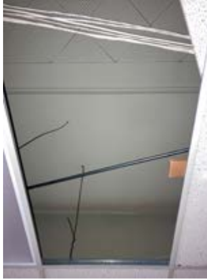
Original ceiling condition.
