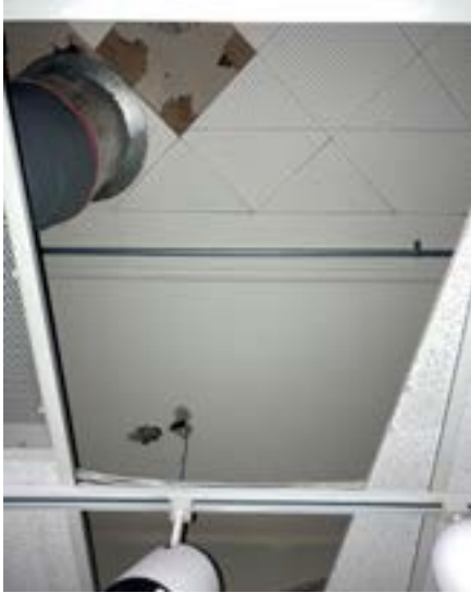
Original ceiling condition.
