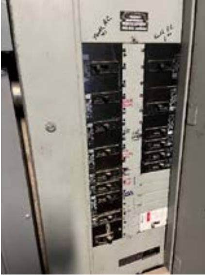
Existing 3 phase, 120/240V high leg panel
