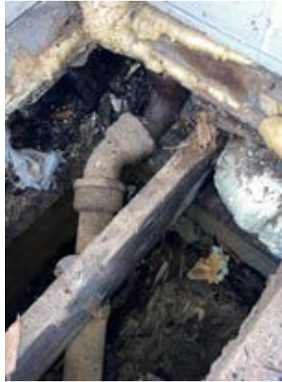
Subfloor condition at northwest corner.
