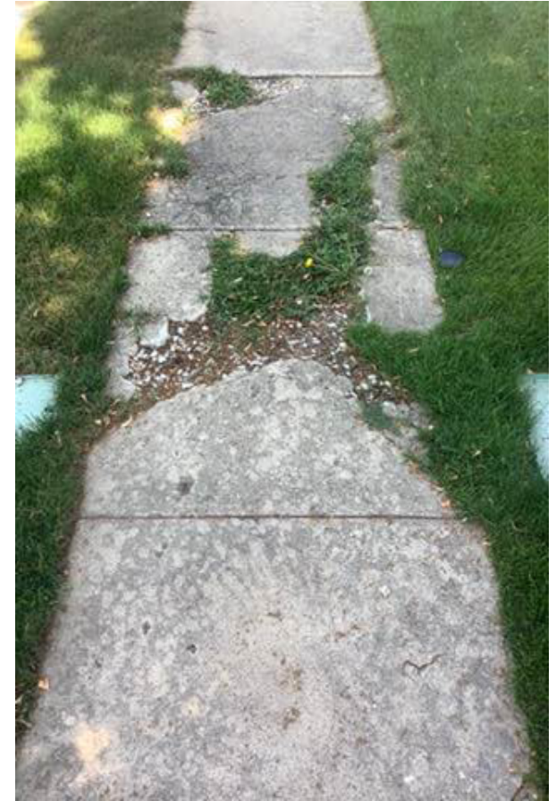
#198 442 N 250 E Cracked Panel
