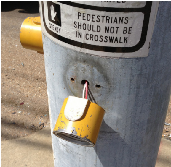
Push-buttons will require regular inspection
